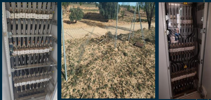
Requena – Copper Cables Theft
